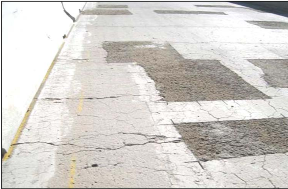
Figure 1: Damage in a Bridge Deck
