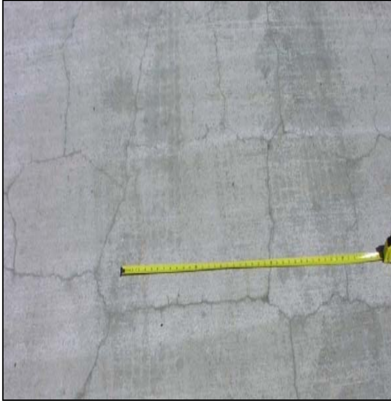
Figure 2: Deck with minor cracking
