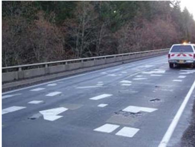
BR2071A: Damage on Deck of Span 1
