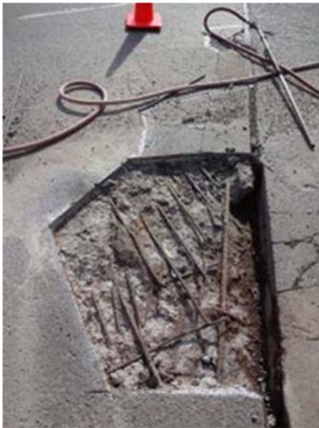
BR09259 Repair Area at Deck-Impact Panel Joint
