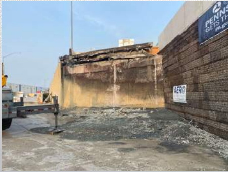
Fire Damaged Abutment 4
